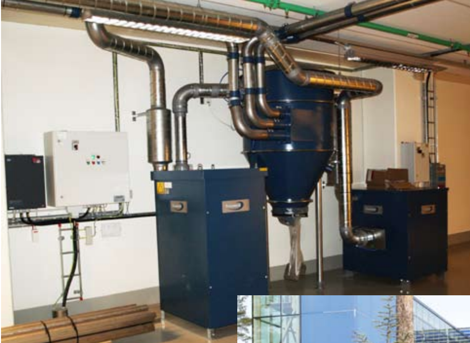
Picture: A stationary vacuum system with Green System is installed in "Satelliten", Absolut Company's new facility outside Åhus in Sweden.
